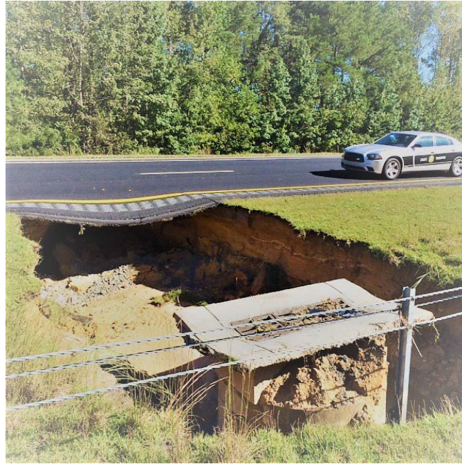
FIGURE 5.12: SINKHOLE IN NORTH CAROLINA
